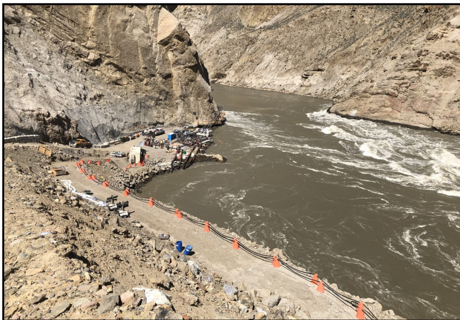
TOP: Crews adjusted the elevation of the Whooshh™ discharge tubes. BOTTOM: View of West Beach work area on July 18.
